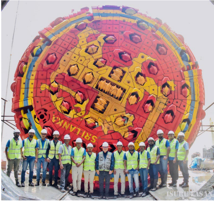
Figure 1: A Team of the project in front of the TBM machine before the commencement of excavation
